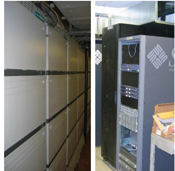
Nortel TDM Telephone Switch and Data Center Server Cabinets (Partial View)
