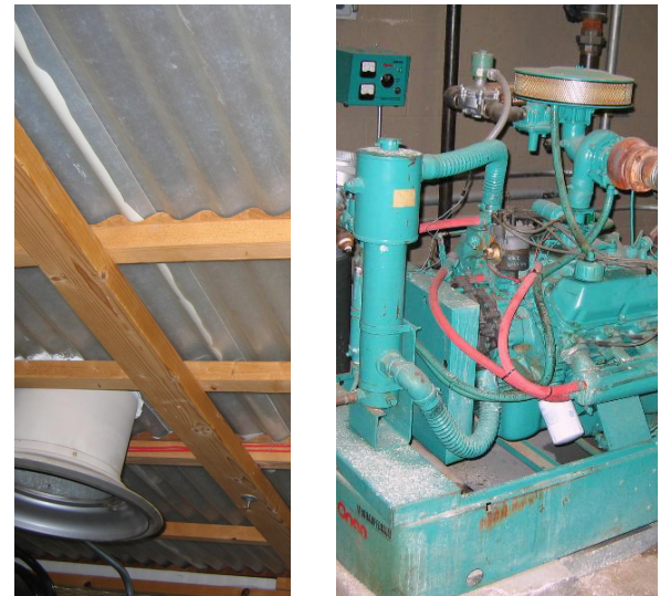
Corrugated Ceiling of Switchgear Room and Emergency Generator (serving Telecom Switchgear Rm)
